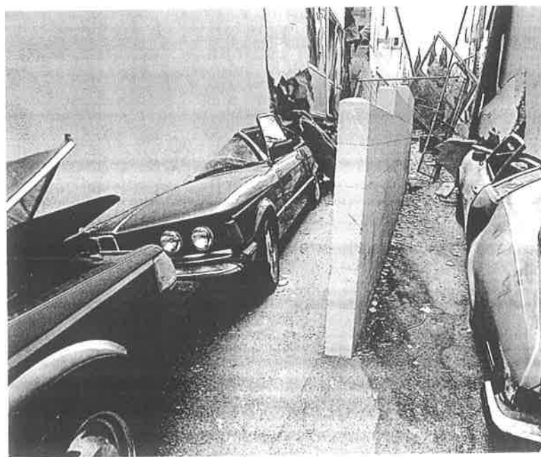
Figure 13 An earthquake shook the ground floor out from under the second story of this apartment building, which then collapsed.
